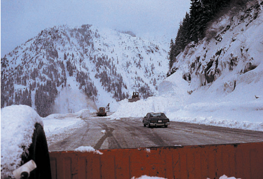
FIGURE 4-4 Removal of avalanche debris along US-2 in Washington. SOURCE: Northwest Weather and Avalanche Center, Seattle, Washington.
